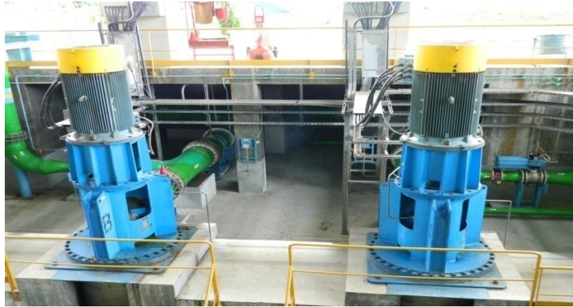
Gambar 2.18 Main Cooling Water Pump Unit 1 PLTP Lahendong
