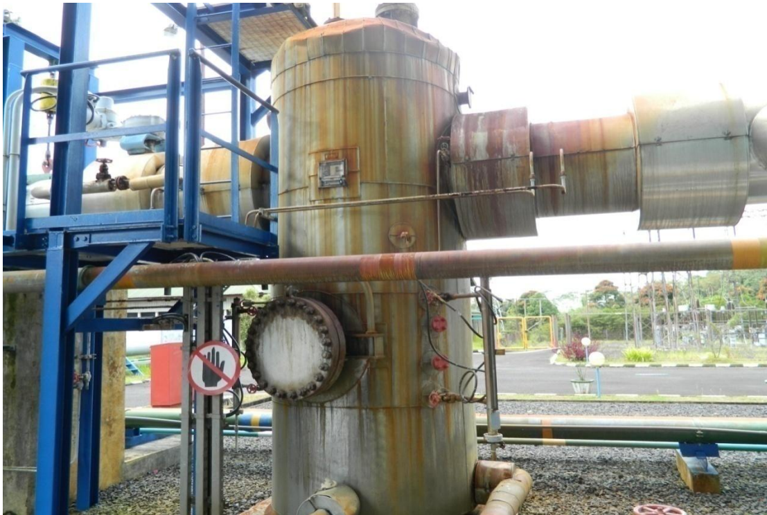
Gambar 2.6 Demister unit 1 PLTP Lahendong
