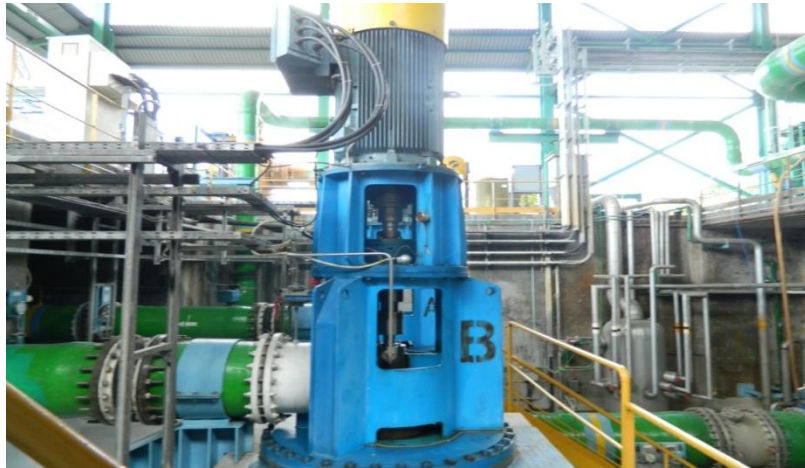
Gambar 2.21 Main Cooling Water Pump B
