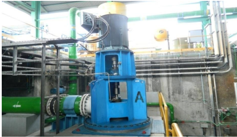
Gambar 2.19 Main Cooling Water Pump A
