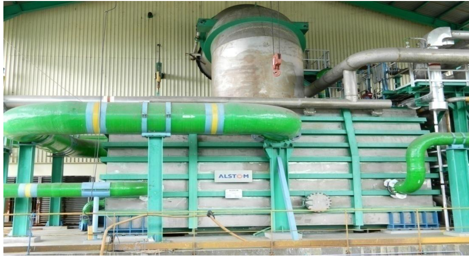
Gambar 2.16 Main Condenser Unit 1 PLTP Lahendong
