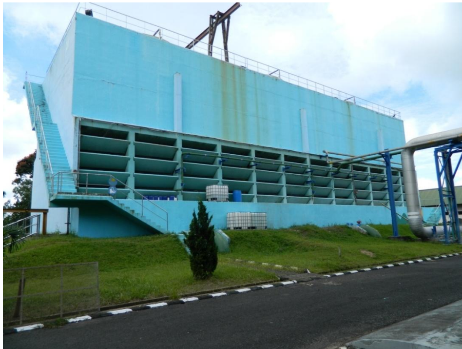
Gambar 2.23 Cooling Tower Unit 1 PLTP Lahendong
