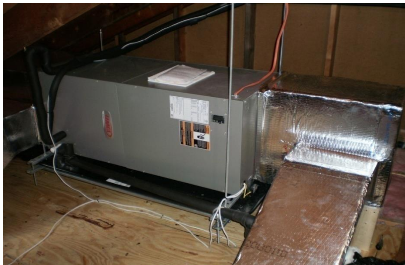
Gambar 4. AC Central unit Indoor
