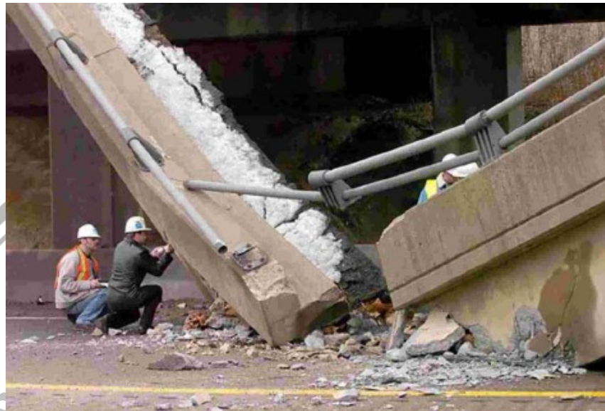
FIGURE 3 Span 3 failure from the Lake View Drive Bridge [2].
