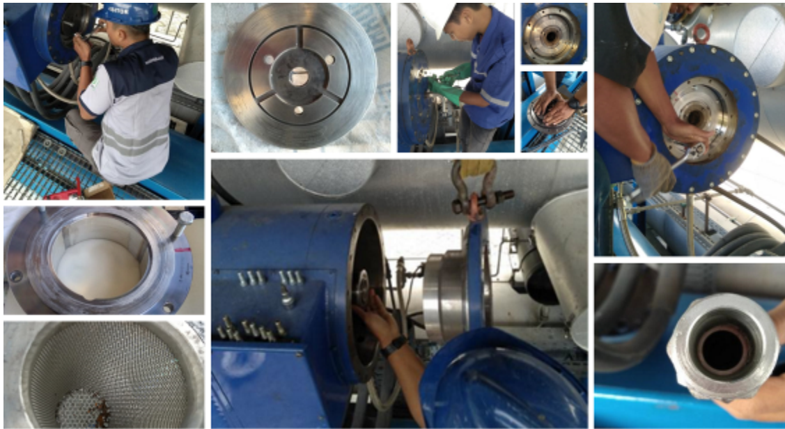
Gambar 3. Kegiatan operation & maintenance PLTP BC 500 kW
