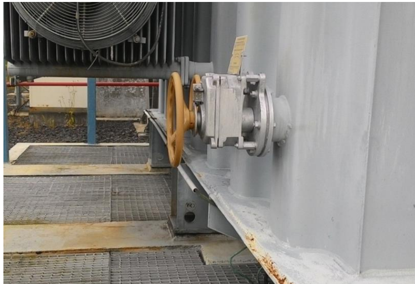
Gambar 3.8. Tap Changer manual Transformator UNINDO PLTP Lahendong.
