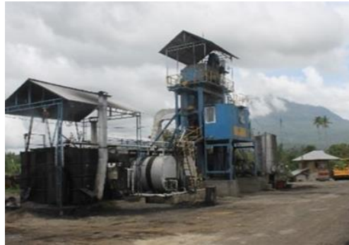
Gambar 2. 1 Asphalt Mixing Plant
