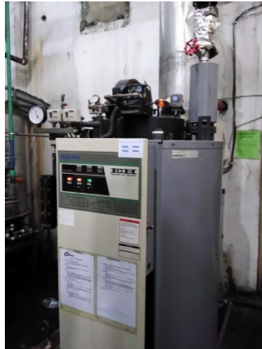
GAMBAR 2.7 Boiler Miura type EH 500 F
